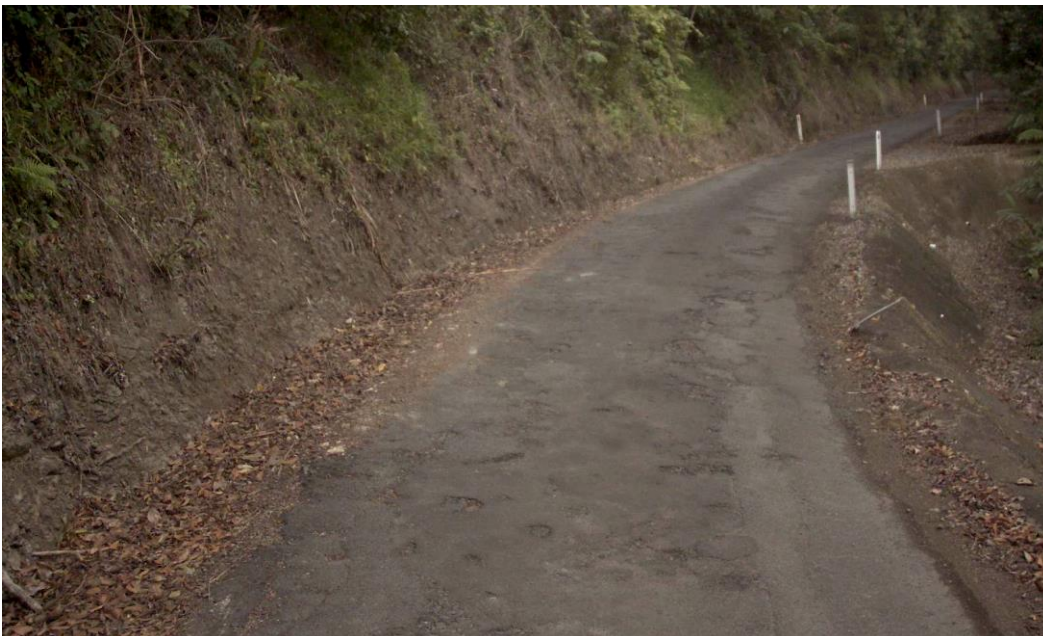
Figure 5.2: Poor surface condition on the Old Palmerston Highway
